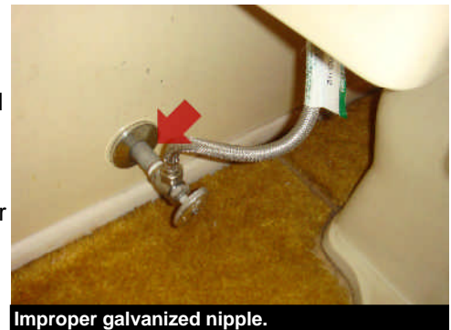
Improper galvanized nipple.
