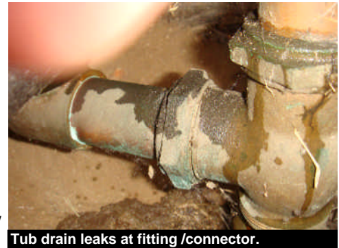
Tub drain leaks at fitting /connector.
