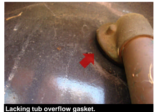
Lacking tub overflow gasket.
