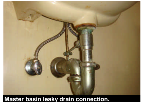
Master basin leaky drain connection.
