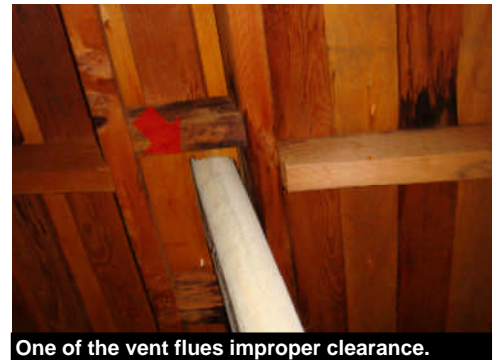
One of the vent flues improper clearance.
