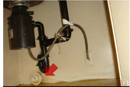
Drain clean-out is provided below sink.
